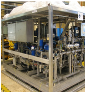
Chemical Injection Unit (CIU)
